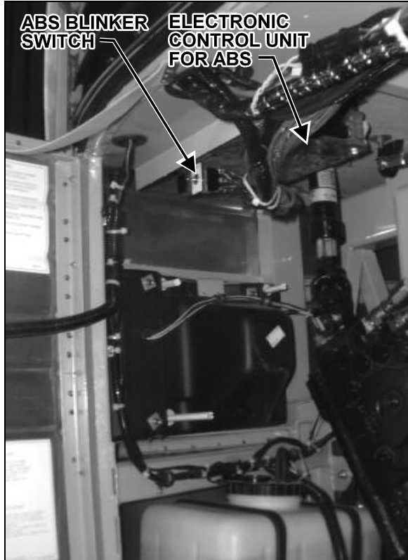
FIGURE 23: STEERING COMPARTMENT (LEFT WALL) 06119
