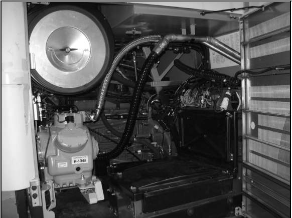
FIGURE 5: REAR ELECTRICAL PANEL, JUNCTION PANEL & BATTERY COMPARTMENT
