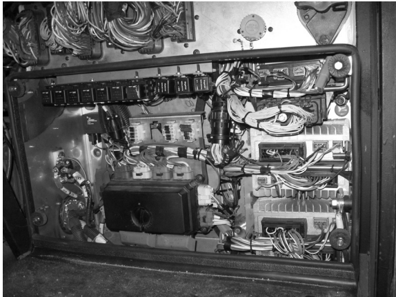
FIGURE 7: REAR ELECTRICAL PANEL
