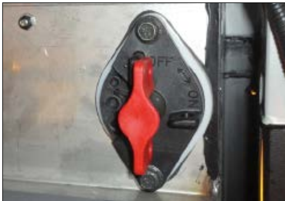
BATTERY MASTER SWITCH
