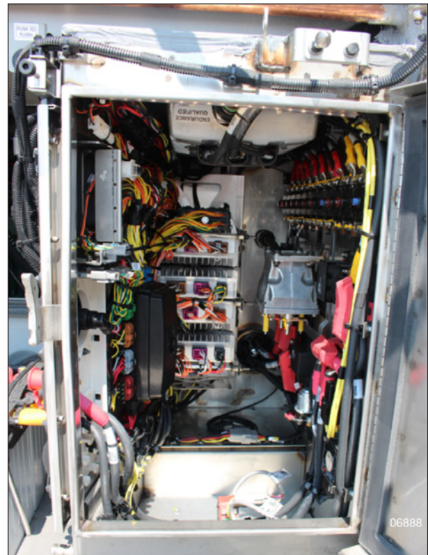
MAIN POWER COMPARTMENT
