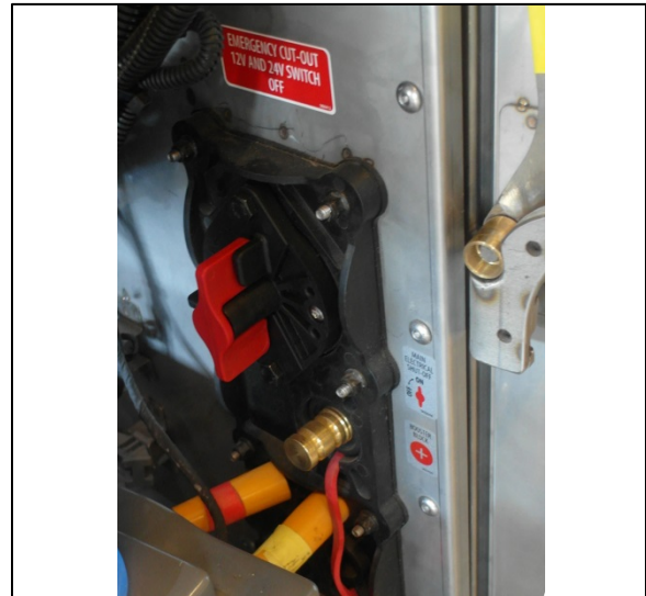
BATTERY MASTER SWITCH
