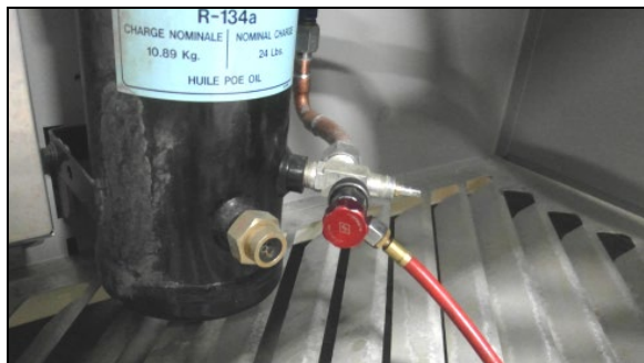
FIGURE 98: RECOVERY UNIT CONNECTED TO RECEIVER SERVICE PORT
