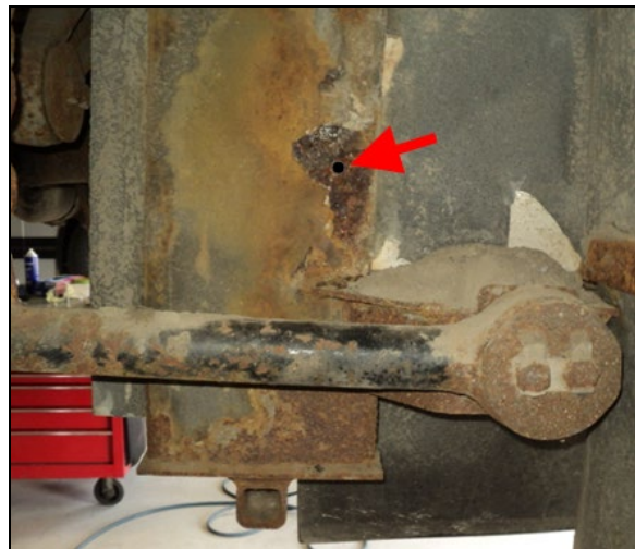
FIGURE 7: HOLE DRILLED IN STRUCTURAL MEMBER
