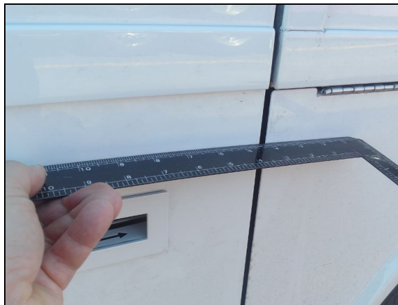
FIGURE 66: USE A RULER (SHOWN IN BLACK) TO CHECK THAT SURFACES ARE EVEN
