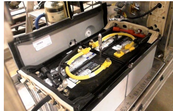
FIGURE 47: BATTERY BANK COVER REMOVED
