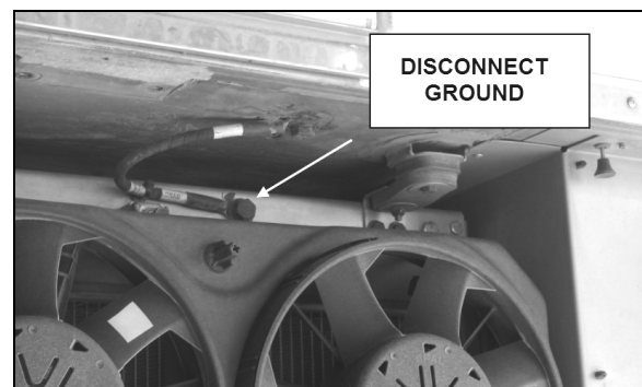
FIGURE 32: COOLING ASSEMBLY GROUND
