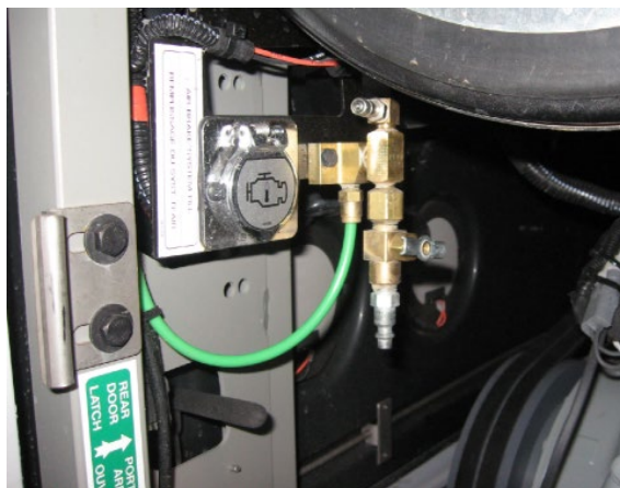
FIGURE 23 : ENGINE COMPARTMENT EMERGENCY AIR-FILL VALVE
