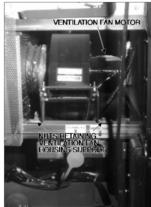
FIGURE 23: VENTILATION FAN MOTOR
