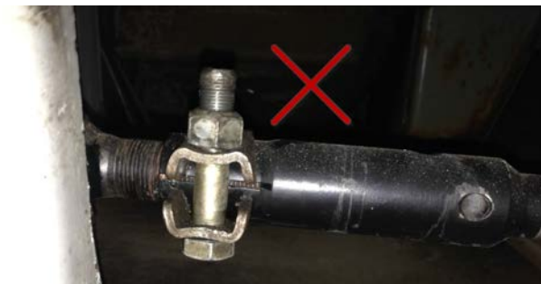
Clamp is bent. Replace clamp.
