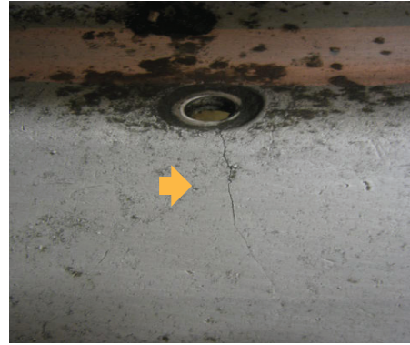
Valve hole crack
