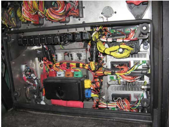
FIGURE 9: REAR ELECTRICAL PANEL
