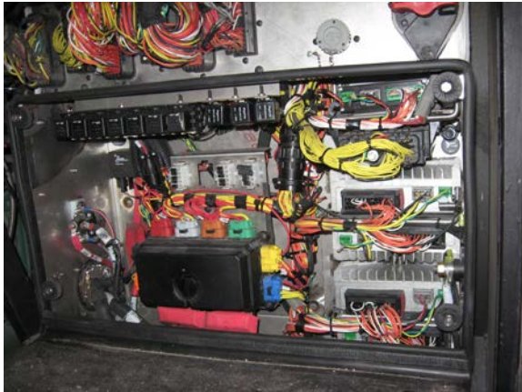
FIGURE 9: REAR ELECTRICAL PANEL
