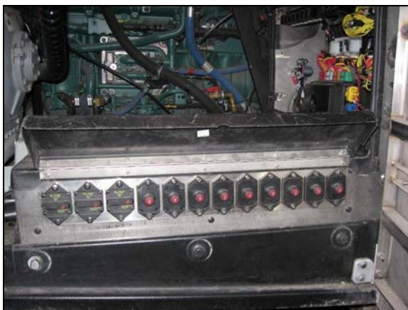
FIGURE 10: REAR ELECTRICAL JUNCTION PANEL 06634
