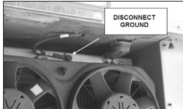
FIGURE 25: COOLING ASSEMBLY GROUND
