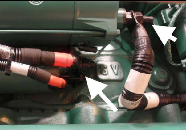
Figure 26: Starter power cable and ground cable lugs protected with Color Guard rubber coating.
