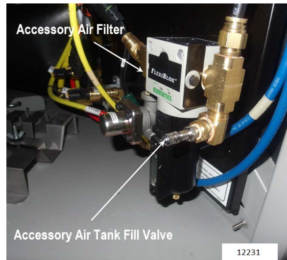
FIGURE 3: FRONT SERVICE COMPARTMENT
