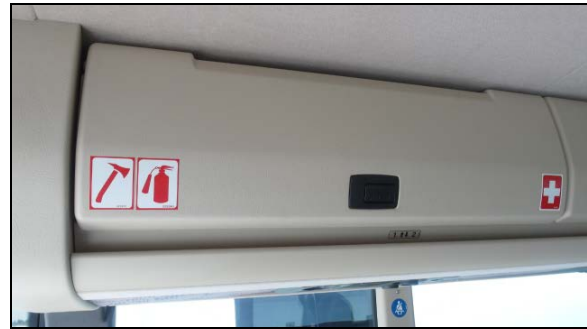
A DECAL INDICATES THAT A FIRE HATCHET, A FIRE EXTINGUISHER AND A FIRST-AID KIT ARE LOCATED IN THIS OVERHEAD COMPARTMENT
