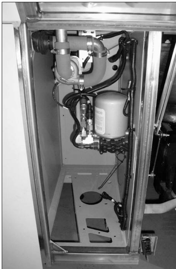
COOLANT HEATER COMPARTMENT
