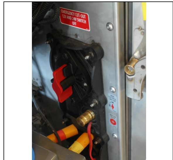
BATTERY MASTER SWITCH
