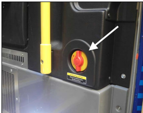
INTERIOR EMERGENCY RELEASE AIR VALVE 12164
