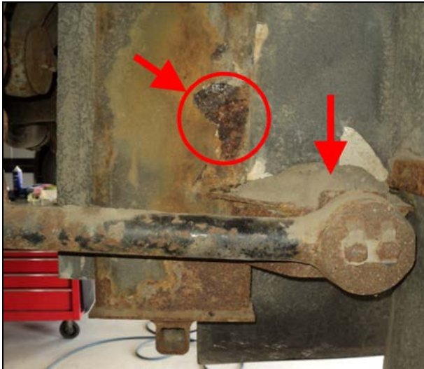
FIGURE 2: METAL FLAKING. ACCUMULATED SAND AS SHOWN ON THE IMAGE SHOULD NOT BE LEFT IN PLACE
