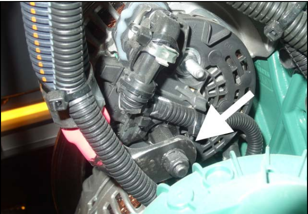
Figure 24: Upper alternator power cable lug protected with Color Guard rubber coating.
