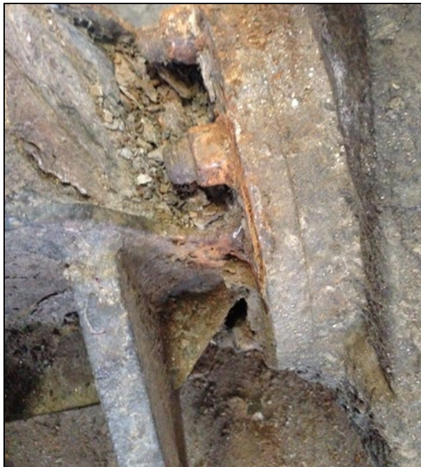
FIGURE 4: METAL FLAKING ON TAG AXLE - ACCUMULATED MATTER WILL RETAIN WATER THUS CREATING CONDITIONS PROMOTING ADDITIONAL CORROSION
