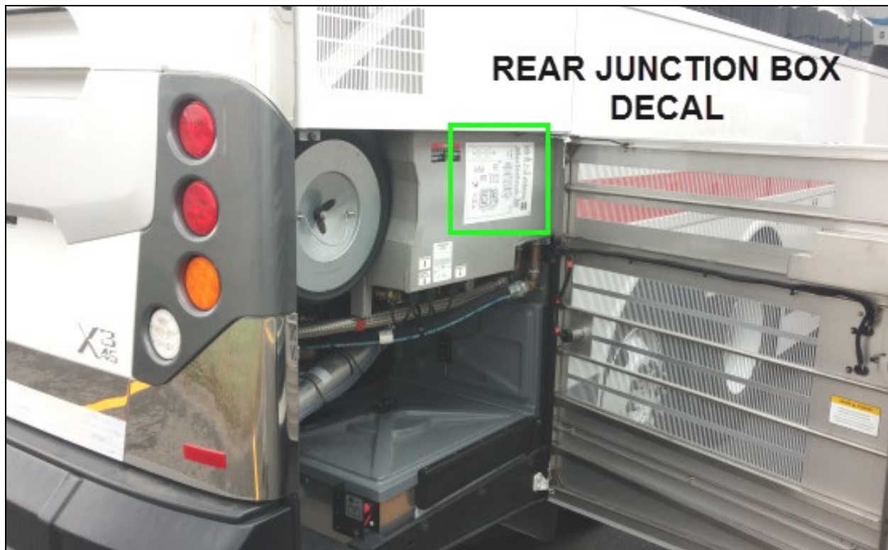
Fig.1 Typical Rear Junction Box localisation in engine compartment (X3 Coach shown)
