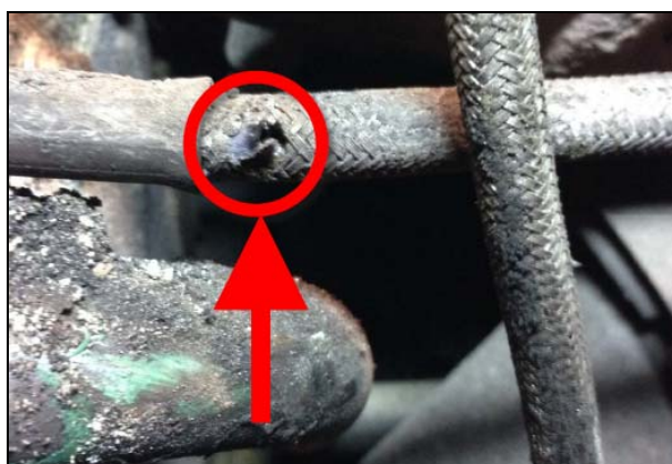
FIGURE 7: EXAMPLE OF DAMAGE ON THE HARD FUEL LINE BRAIDED SECTION CAUSED BY THE AIR PURGE LINE
