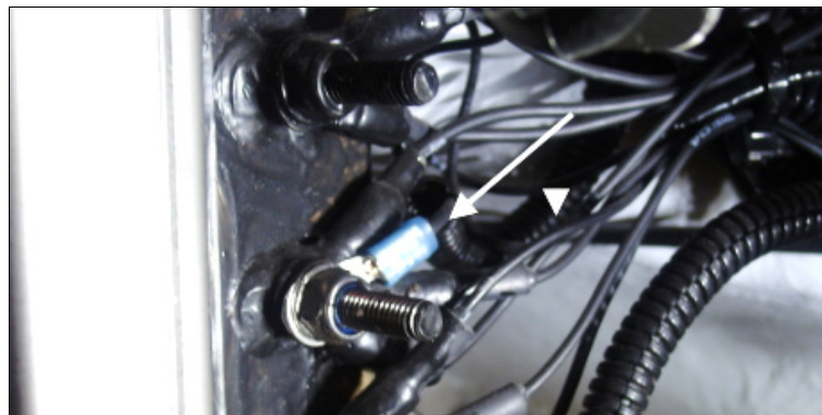
GROUND WIRE CONNECTED
