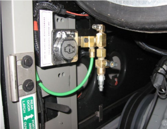
FIGURE 23 : ENGINE COMPARTMENT EMERGENCY AIR-FILL VALVE
