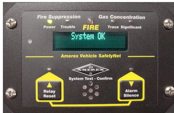
Figure 4.6.1e—Indicates all connected components are OK
