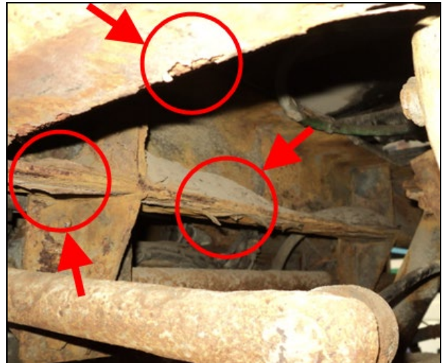
FIGURE 3: METAL FLAKING AND ACCUMULATED SAND
