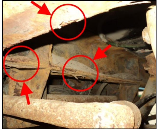
FIGURE 3: METAL FLAKING AND ACCUMULATED SAND
