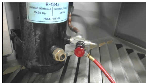
FIGURE 100: RECOVERY UNIT CONNECTED TO RECEIVER SERVICE PORT
