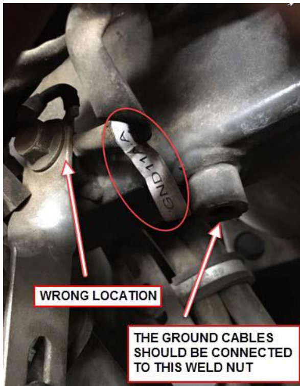
FIGURE 3: WRONG CONNECTION OF GROUND CABLES
