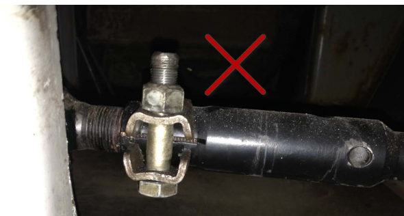
Clamp is bent. Replace clamp.
