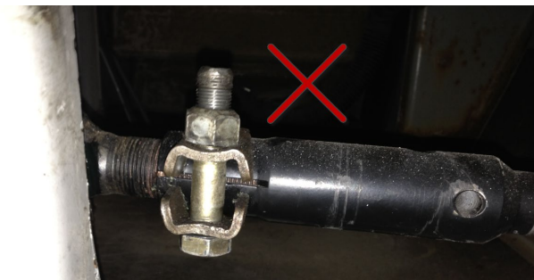
Clamp is bent. Replace clamp.
