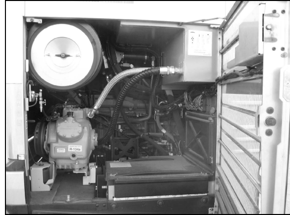
ENGINE COMPARTMENT R.H. SIDE 18607
