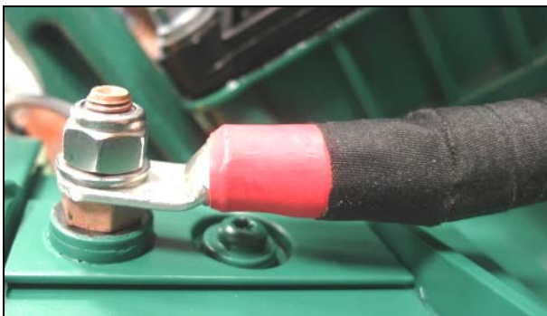
Figure 16: No exposed or broken copper strands.
