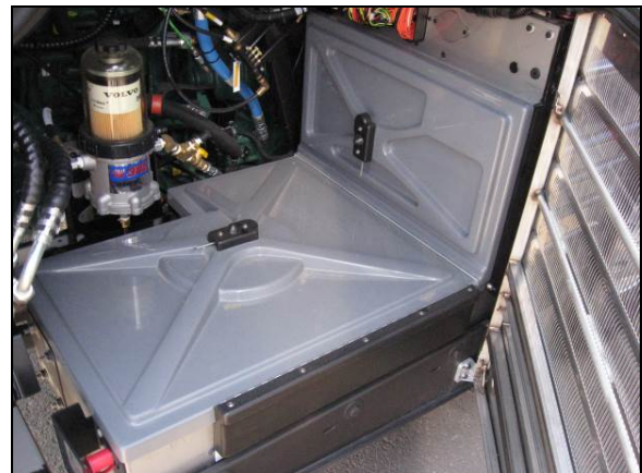
FIGURE 8: REAR ELECTRICAL PANEL, JUNCTION PANEL & BATTERY COMPARTMENT
