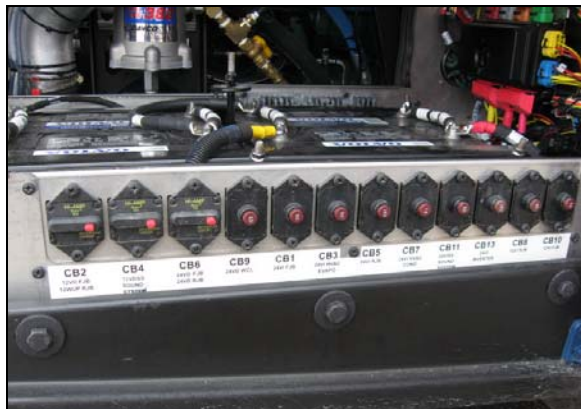
FIGURE 11: REAR ELECTRICAL JUNCTION PANEL
