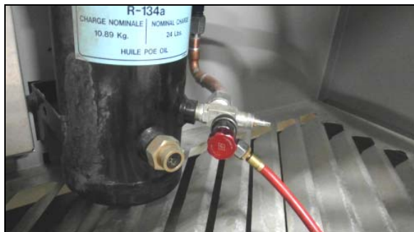
FIGURE 80: RECOVERY UNIT CONNECTED TO RECEIVER SERVICE PORT
