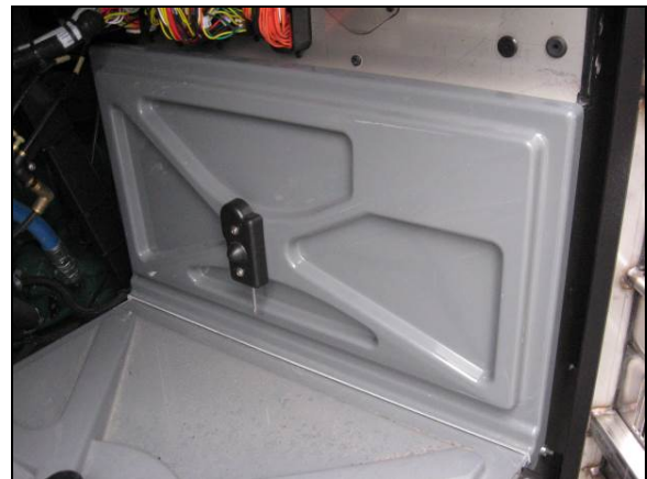
FIGURE 9: REAR ELECTRICAL PANEL
