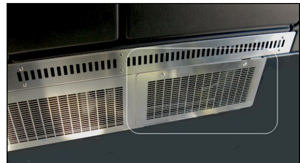
ACCESS TO DRIVER'S HVAC UNIT AIR FILTERS
