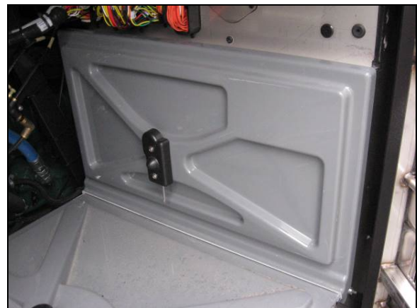
FIGURE 9: REAR ELECTRICAL PANEL
