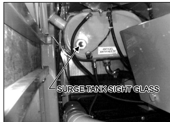
FIGURE 4: SURGE TANK SIGHT GLASS 05038
