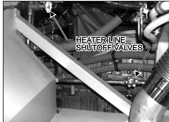
FIGURE 39: HEATER LINE SHUTOFF VALVES WITHOUT PREHEATER 05041
