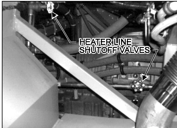
FIGURE 7: HEATER LINE SHUTOFF VALVES 05041
