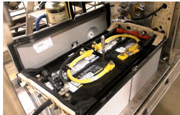
FIGURE 42: BATTERY BANK COVER REMOVED
