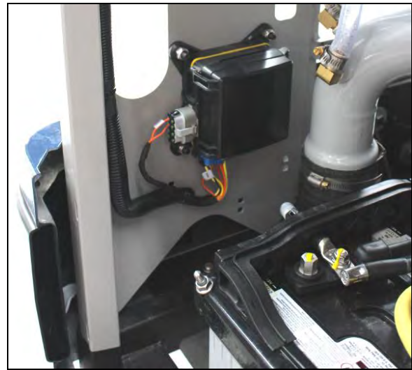
FIGURE 46: VECT (CURB SIDE)
