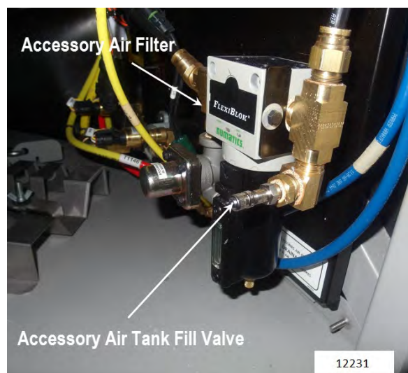
FIGURE 4: FRONT SERVICE COMPARTMENT
