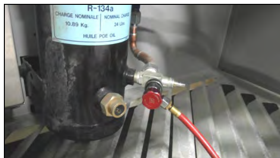
FIGURE 83: RECOVERY UNIT CONNECTED TO RECEIVER SERVICE PORT
