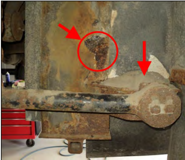
FIGURE 2: METAL FLAKING. ACCUMULATED SAND AS SHOWN ON THE IMAGE SHOULD NOT BE LEFT IN PLACE
