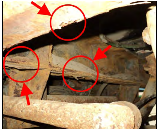
FIGURE 3: METAL FLAKING AND ACCUMULATED SAND
