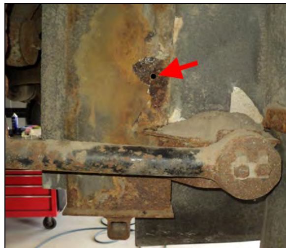
FIGURE 7: HOLE DRILLED IN STRUCTURAL MEMBER
