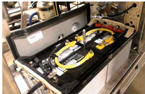
FIGURE 42: BATTERY BANK COVER REMOVED
