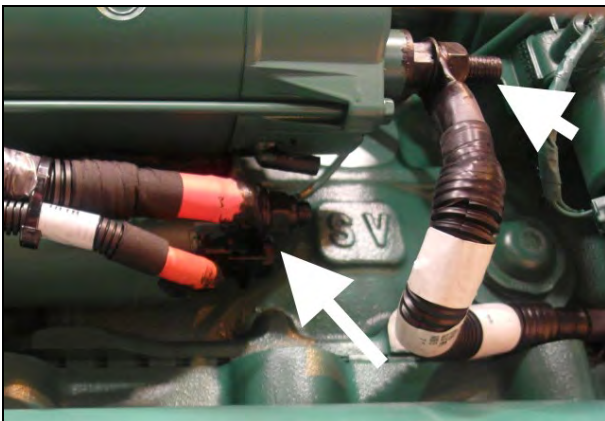
Figure 30: Starter power cable and ground cable lugs protected with Color Guard rubber coating.
