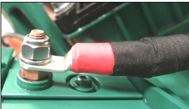
Figure 16: No exposed or broken copper strands.
