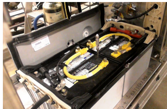
FIGURE 42: BATTERY BANK COVER REMOVED
