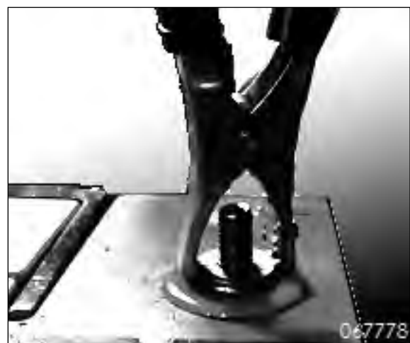
FIGURE 57 ALLIGATOR CLAMP POSITION- TYPICAL AGM BATTERY
