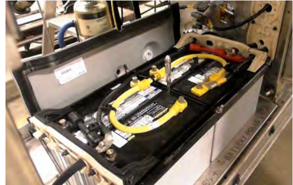
FIGURE 43: BATTERY BANK COVER REMOVED
