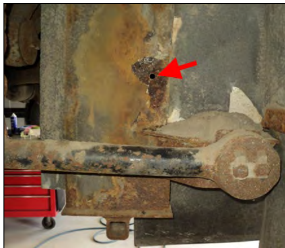
FIGURE 7: HOLE DRILLED IN STRUCTURAL MEMBER
