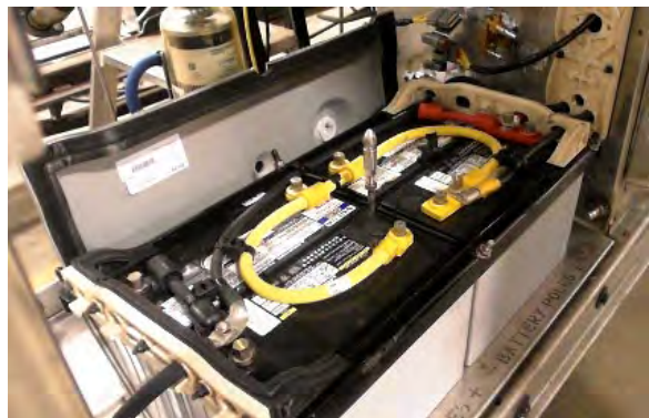
FIGURE 31: BATTERY BANK COVER REMOVED
