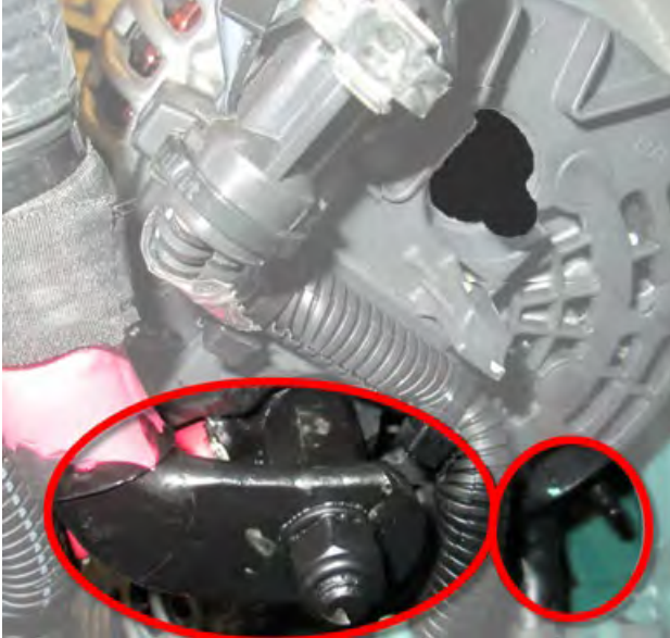
Figure 27: Upper R.H. side Bosch alternator power cable lug protected with Color Guard rubber coating.
