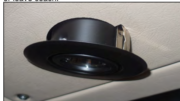
FIGURE 83: DRIVER'S AREA CEILING LIGHT
