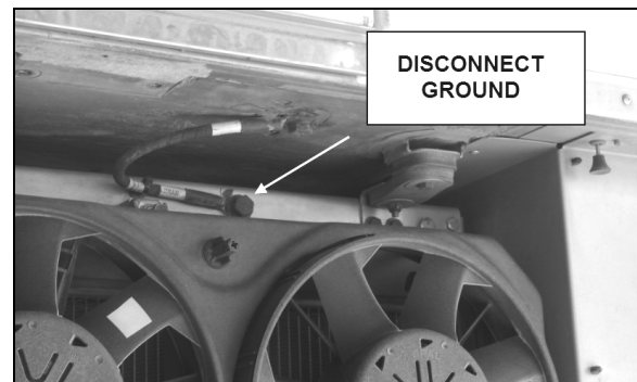
FIGURE 32: COOLING ASSEMBLY GROUND
