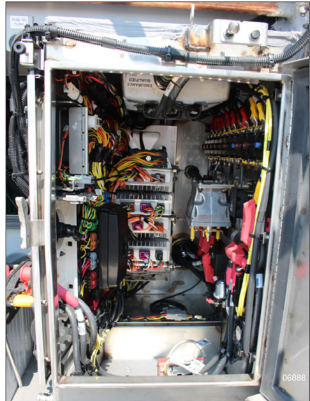
MAIN POWER COMPARTMENT
