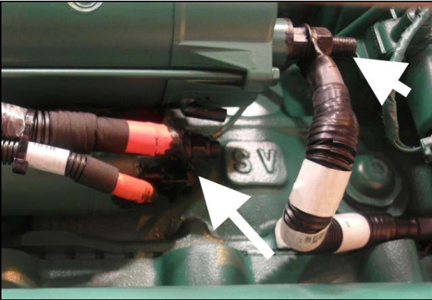
Figure 26: Starter power cable and ground cable lugs protected with Color Guard rubber coating.
