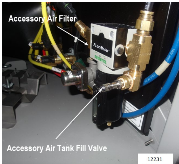
FIGURE 4: FRONT SERVICE COMPARTMENT
