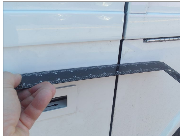
FIGURE 66: USE A RULER (SHOWN IN BLACK) TO CHECK THAT SURFACES ARE EVEN
