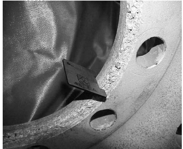
Hub bore gauge with severe corrosion. Remove any severely corroded wheel from service
