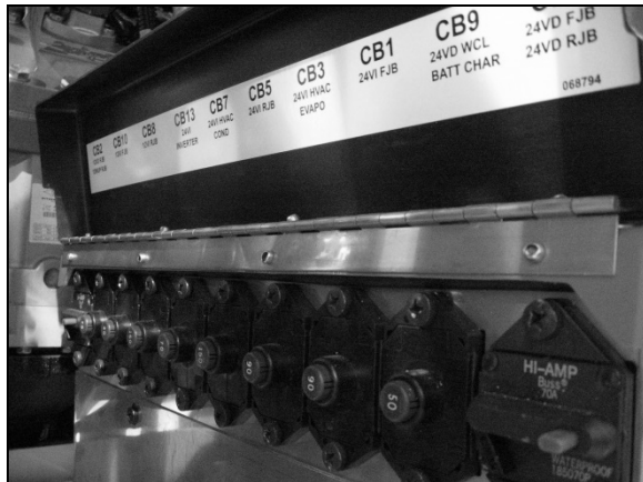
Figure 2: Circuit Breaker Panel 06621
