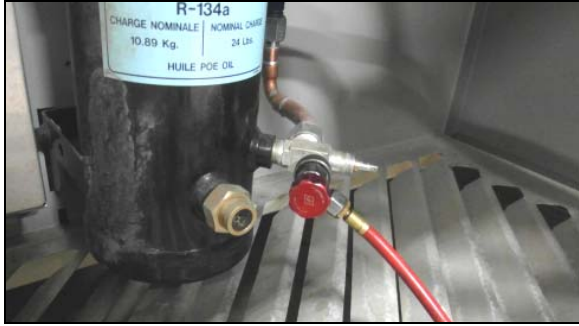
FIGURE 22: RECOVERY UNIT CONNECTED TO RECEIVER SERVICE PORT
