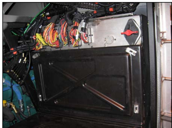
FIGURE 8: REAR ELECTRICAL PANEL
