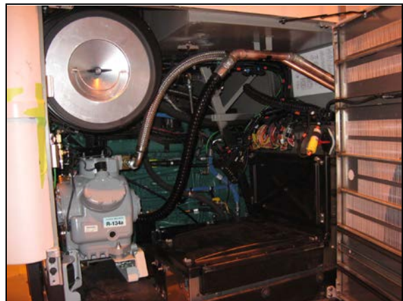
FIGURE 7: REAR ELECTRICAL PANEL, JUNCTION PANEL & BATTERY COMPARTMENT
