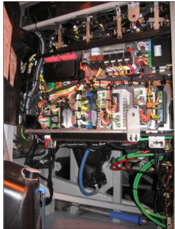
FRONT SERVICE COMPARTMENT
