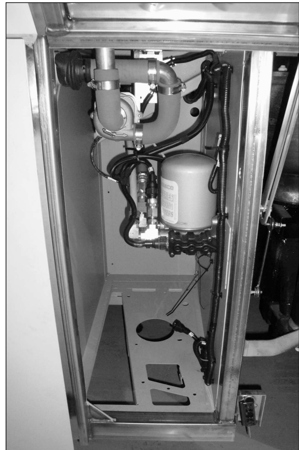
COOLANT HEATER COMPARTMENT
