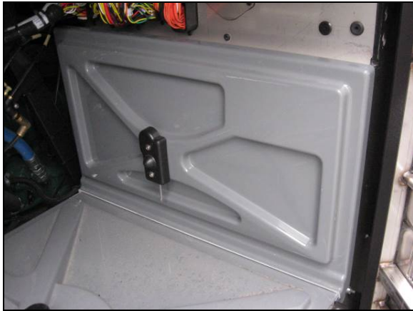
FIGURE 9: REAR ELECTRICAL PANEL
