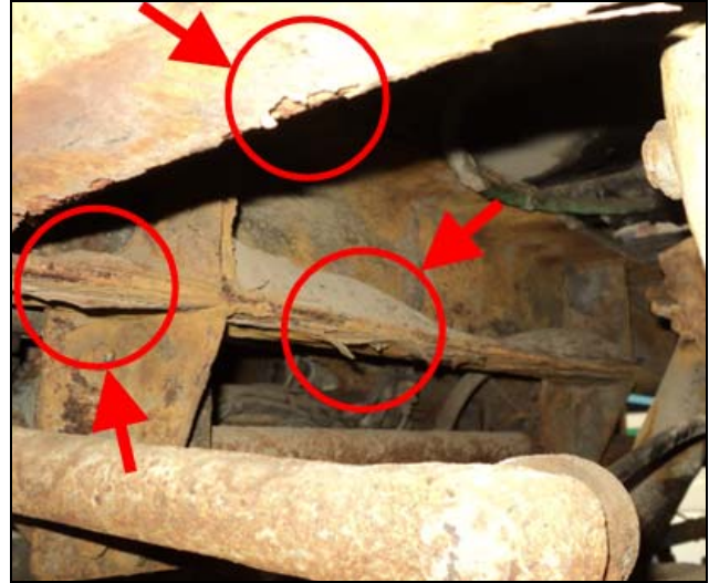
FIGURE 3: METAL FLAKING AND ACCUMULATED SAND
