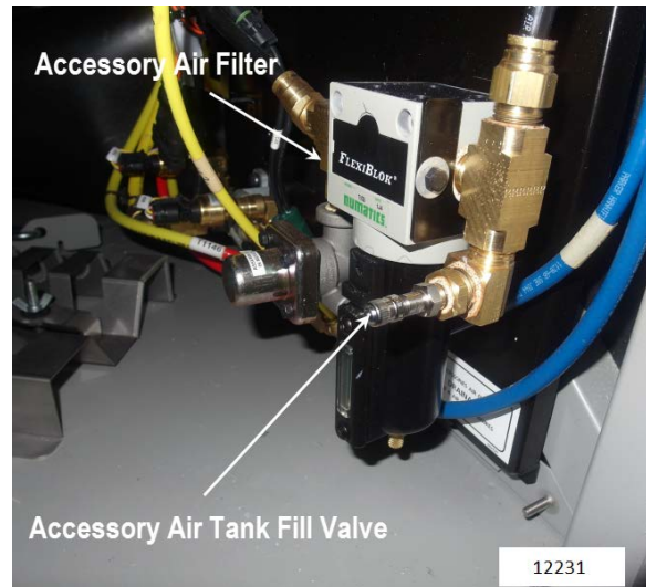
FIGURE 3: FRONT SERVICE COMPARTMENT
