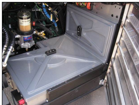
FIGURE 8: REAR ELECTRICAL PANEL, JUNCTION PANEL & BATTERY COMPARTMENT
