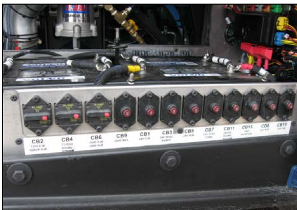
FIGURE 10: REAR ELECTRICAL JUNCTION PANEL
