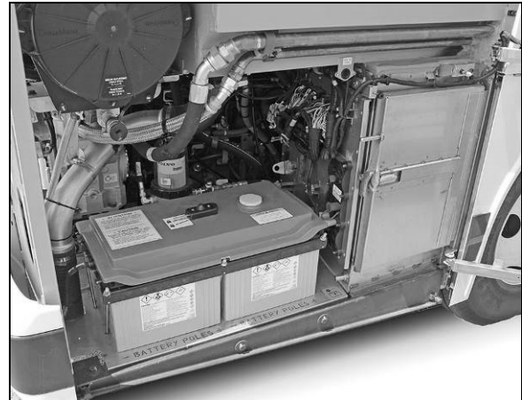
ENGINE COMPARTMENT R.H. SIDE
